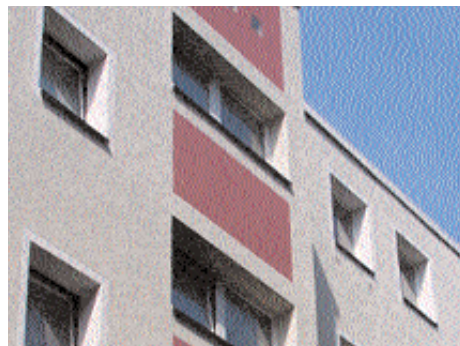
Growth of algae produces green stains on the outside walls of buildings.
